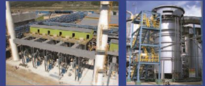
Hot Oil Heater
